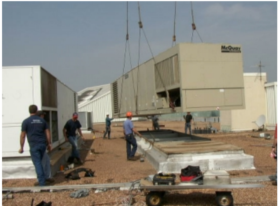
Specified to the exact curb dimensions as the original units, the new modular McQuay rooftop units were installed easily and quickly on a Sunday morning before the mall opened. The old unit pictured at left will also be replaced.
