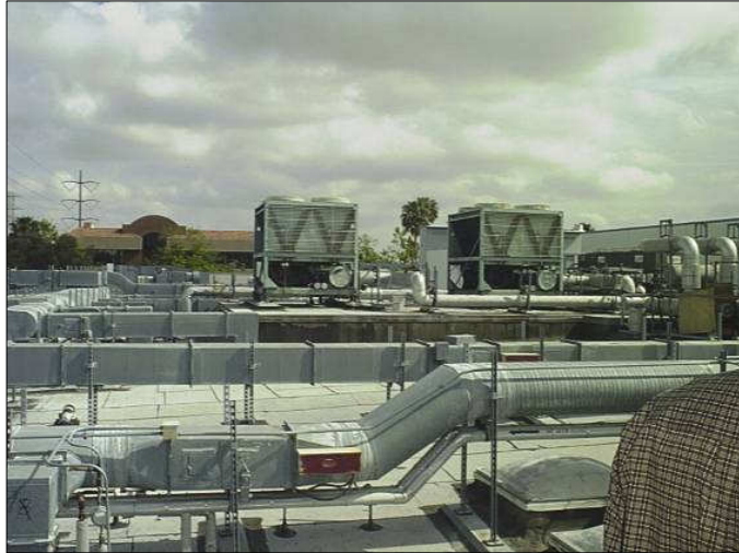
Figure 1: Rooftop ductwork and existing air-cooled chillers.
