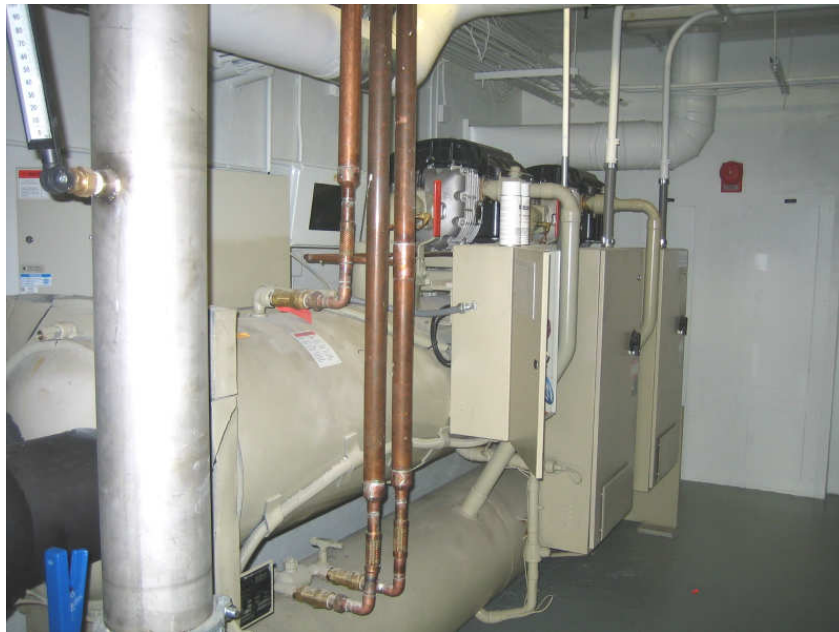
Figure 3: One of the two new WMC150 McQuay Turbocor chillers
