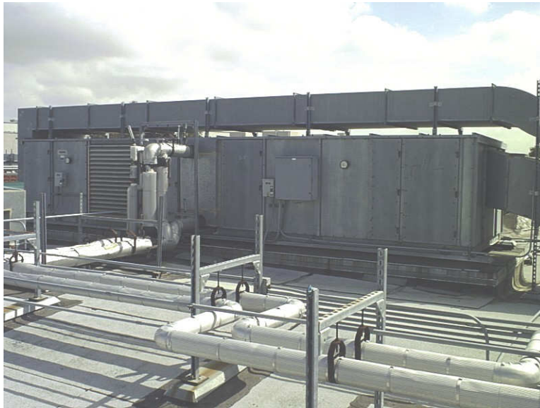
Figure 7: Original VAV air-handler at the Crime Lab
